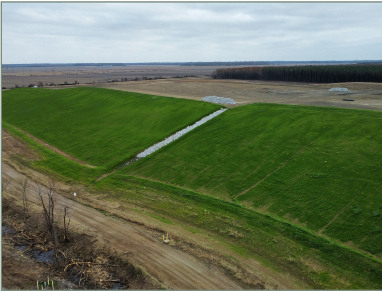
Photo No. 1 Looking south at the north slope active Cell 14 and Cell 15.
