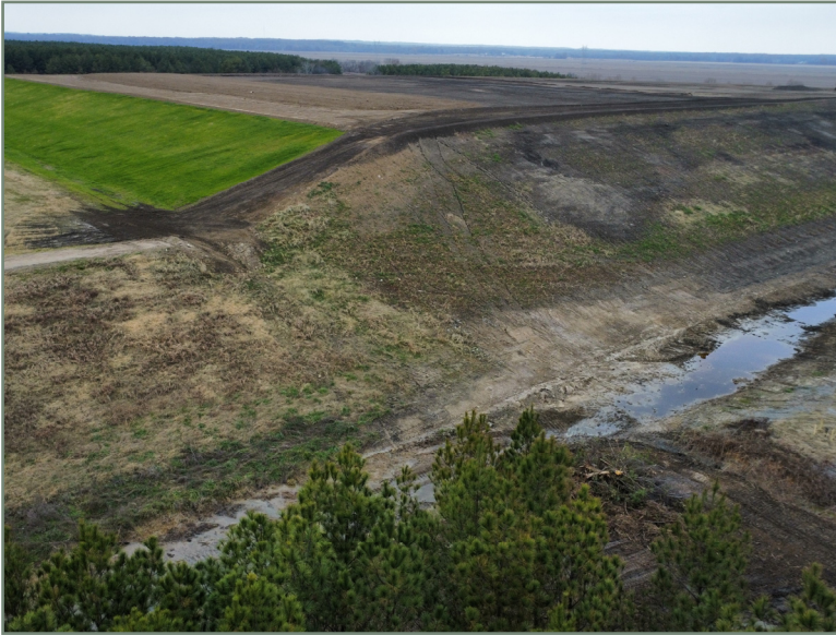
Photo No. 7 Looking north at the north and east slope of active Cell 12.
