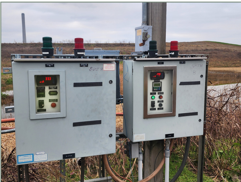
Photo No. 3 Looking west at the leachate control panels for active Cell 15.
