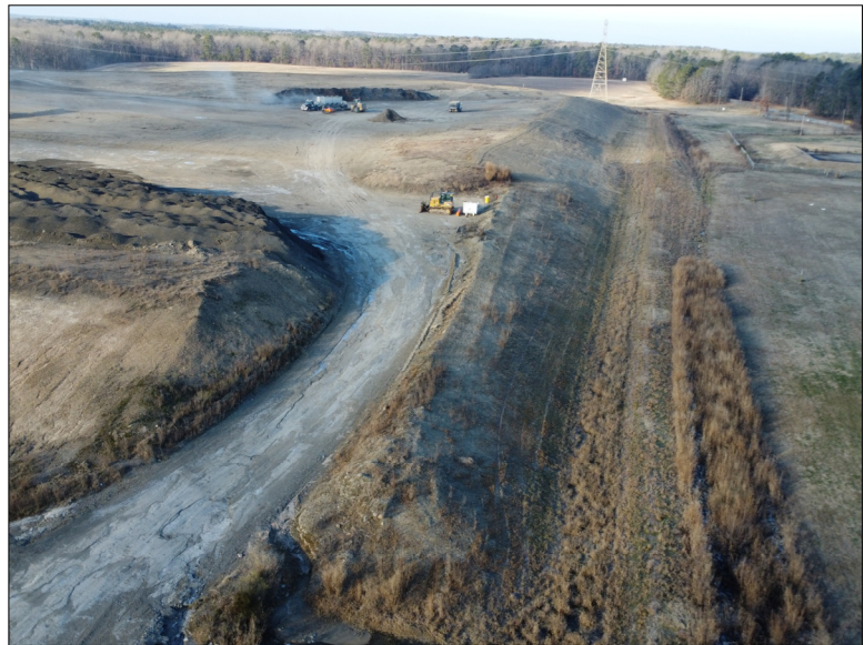
Photo No. 5 Looking west at the north slope of active Cell 1 and Cell 3. The east access road to the top of the Landfill is shown in the foreground.
