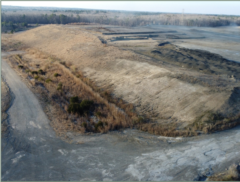
Photo No. 4 Looking south at the east slope of Cell 1 and Cell 2.
