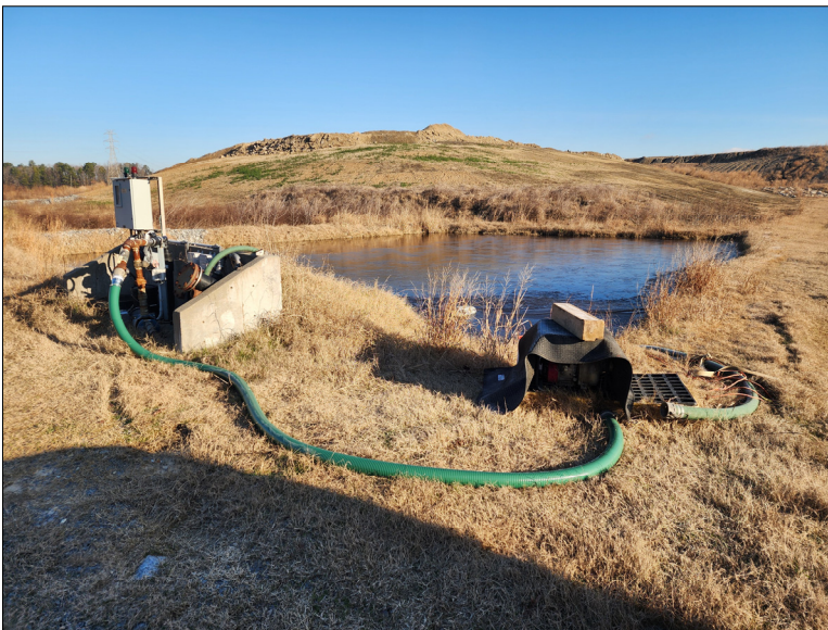
Photo No. 9 Looking north at the leachate collection sump and riser headwall for Active Cell 4.
